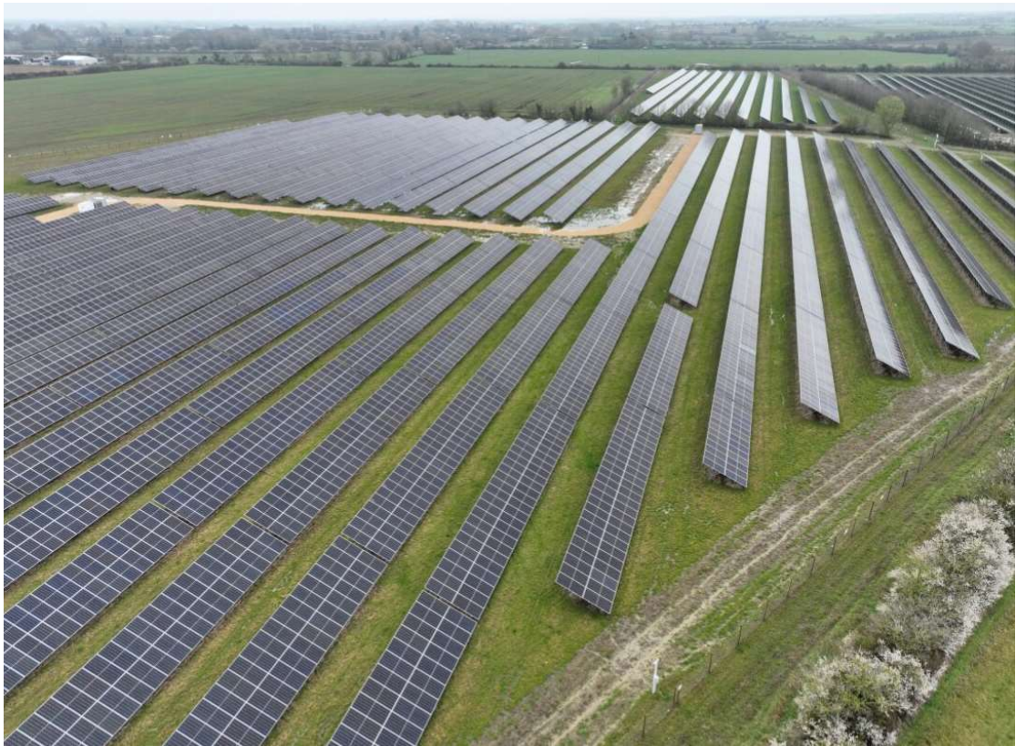
FIGURE 9.1 – EXAMPLE OF SOLAR ARRAYS
